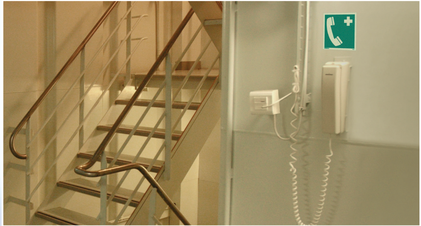
4392C (Emergency telephone)
